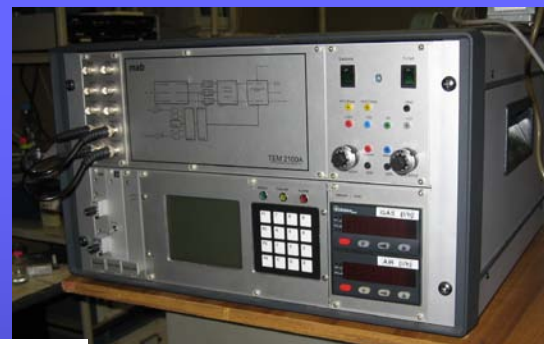
Tritium monitor behind safety wall
