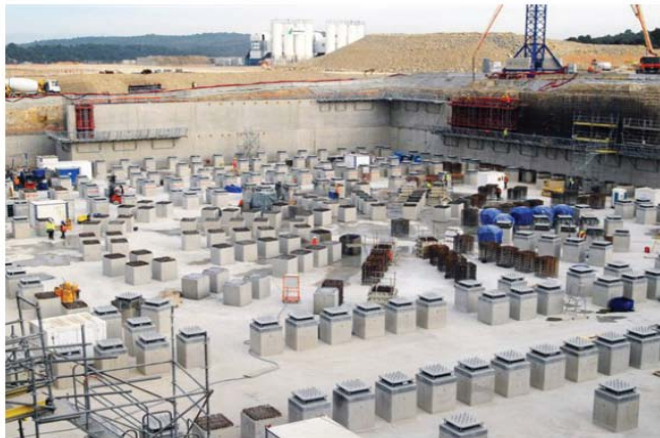
Tokamak complex: 280 plinths and 220 anti-seismic bearings already in place using 700 m 3 of concrete and 300 tonnes of iron. January 2012
